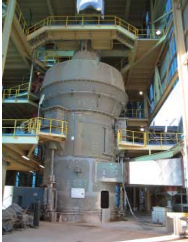
2 MPS 4500 B kurz vor Montageschluss 2 MPS 4500 B shortly before completion of assembly
