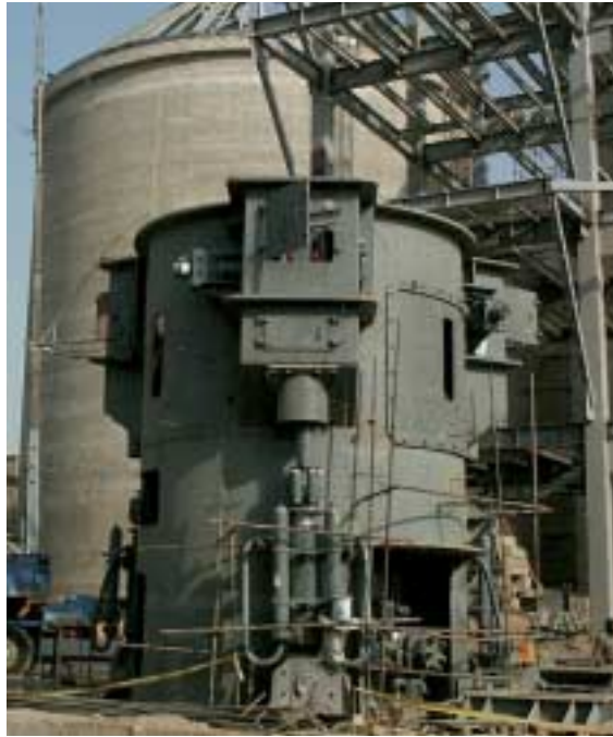
2 Montage einer Zementmühle MPS 4250 BC im Werk Tehran Cement 2 Erection of a finish grinding mill MPS 4250 BC at Tehran Cement
