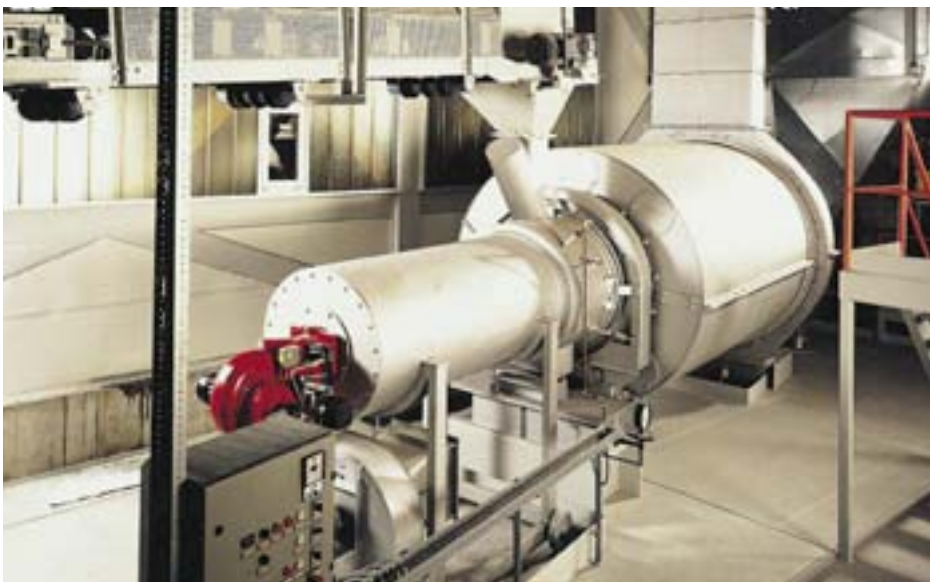
TRT Triplex dryer with hot gas generator
