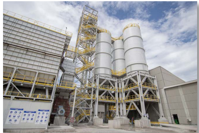
Figure 7: Product silos (B. 1) of the ready2grind plant in Caldera
