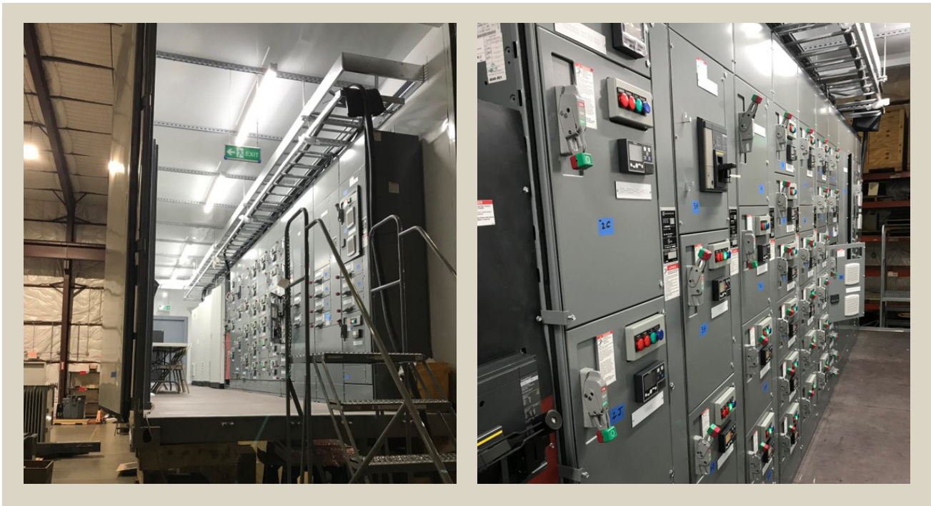
Figure 4: Electrical system, container module (A. 5)
