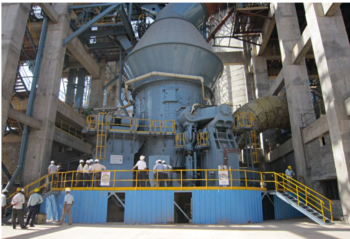
10 The MVR 5600 C-4 at the Balaji plant (India) in June 2012 after commissioning
