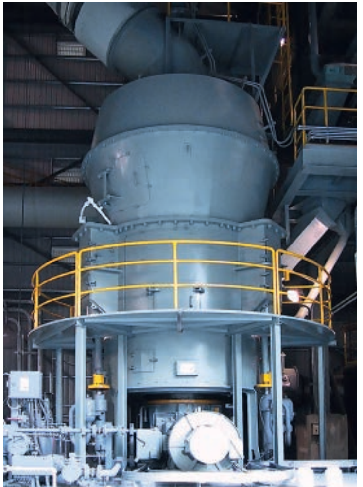
Grinding of limestone with MPS 200 B in Taiwan
